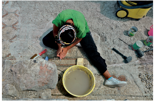
Res. 6 a-b Kilise taban mozaiki ve terrakotta taban döşemesi onarımı, 2011 Fig. 6a-b Repair of floor mosaics and terra cotta flooring at church, 2011
